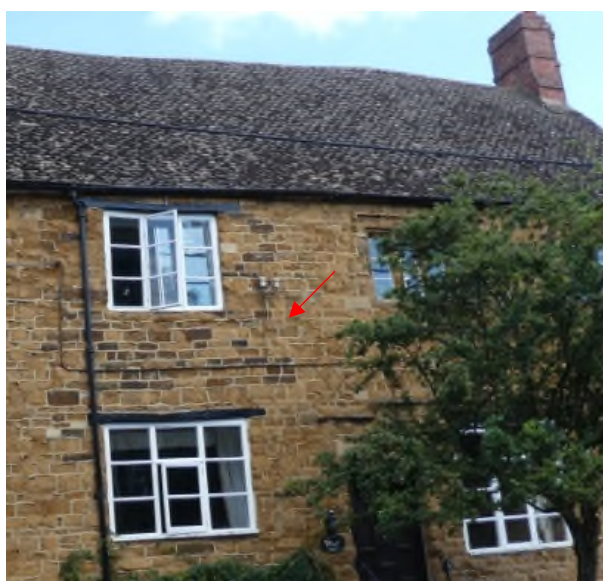
Figure 13: Apparent building break to the left of the front door at Plough House
