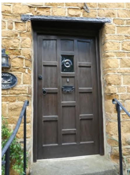
Figure 19: Existing front entrance with a slender timber lintel, no stone dressings and a modern door
