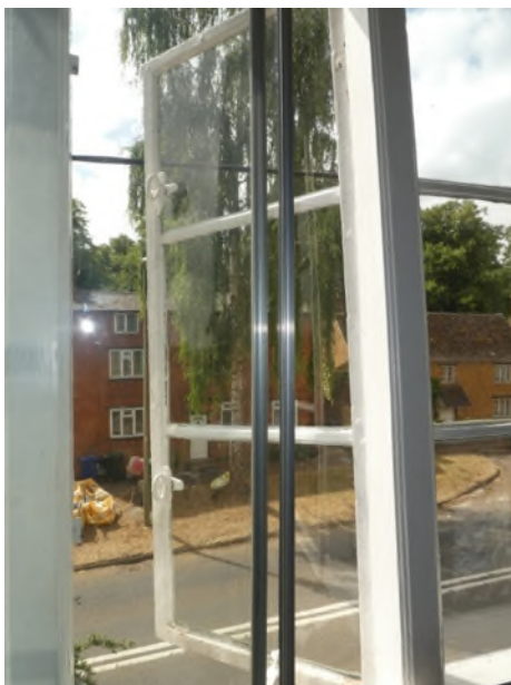
Figure 36: Side opening iron casement with evidence for lead comes on the south-west side of bedroom 1
