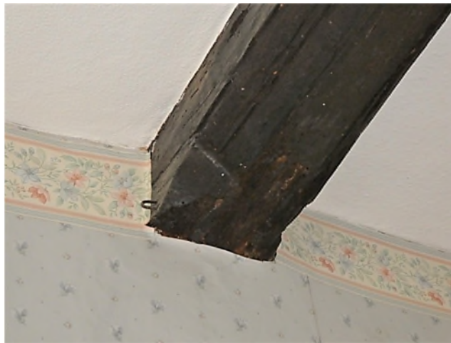
Figure 34: Detail of the double ovolo mouldings and scroll stop on the axial beam in bedroom 1
