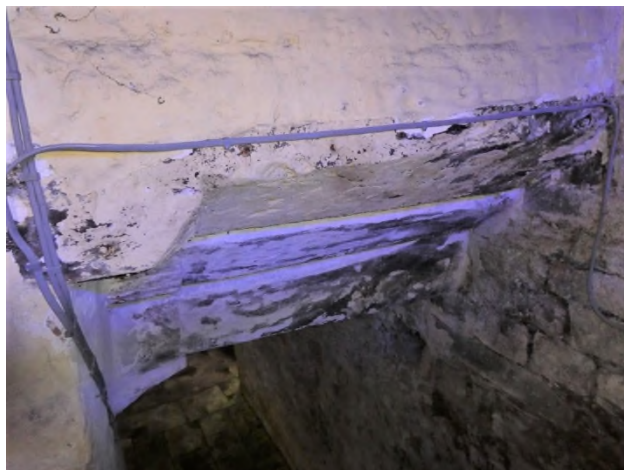
Figure 28: Stone lintel with a wide chamfer and flat-step stops at the entrance to the cellar
