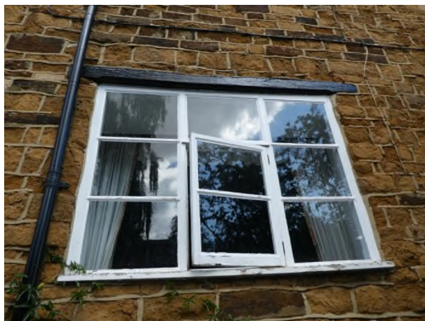
Figure 18: Detail of the ground floor window to the left of the front door
