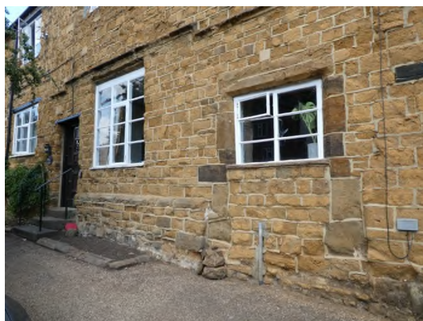
Figure 16: Partially infilled door on the right hand side of the front elevation, string course and modified window opening to the right of the front door
