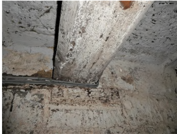
Figure 30: Detail of the wide chamfered axial beam with scroll stops in the cellar
