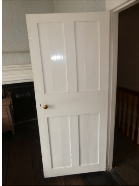
Figure 55: 4-panelled door with plain sunk panels leading from the landing to bedroom 1
