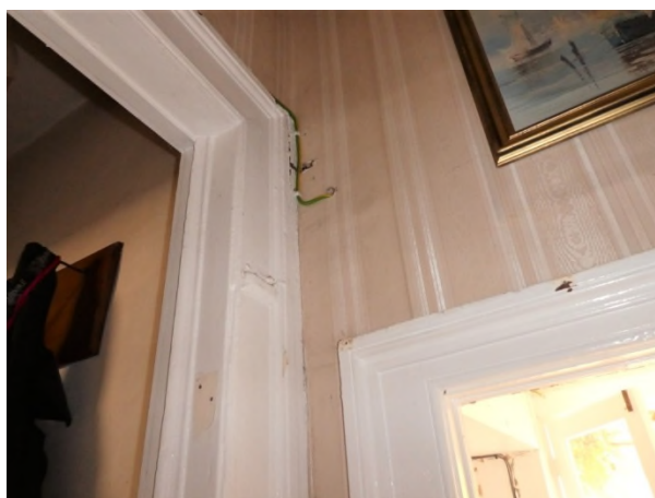
Figure 50: Architraves to the rear door and door to the stairs from the entrance hall
