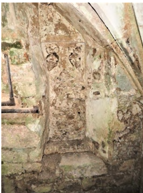
Figure 12: Blocked tracery window
