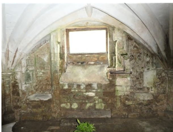
Figure 11: Front wall of the cellar which includes a partially infilled door and blocked windows
